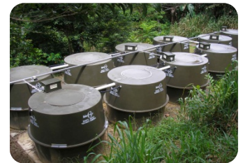
Waste Treatment System
